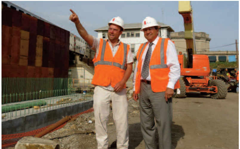
Joliet Mayor Tom Giarrante (right) recently received a progress update on the Joliet Gateway Center from Nick Bostic (left), Project Manager with the Orland Park, IL-based John Burns Construction Company.
